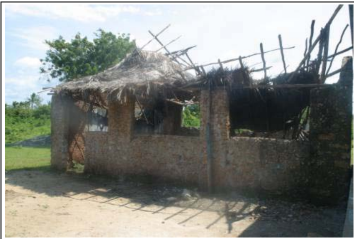
collapsed roof at Bahari Primary School
